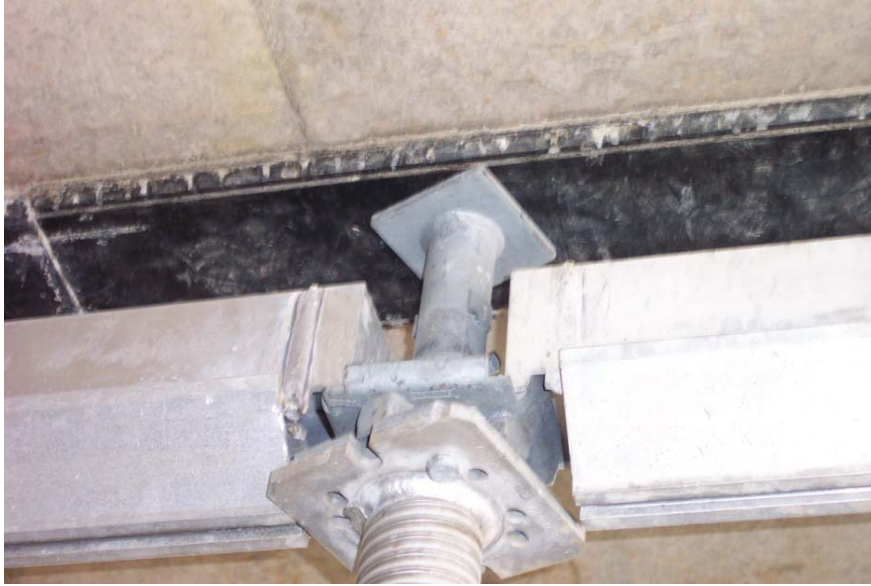
Incorrect Position – Prop/Drophead off centre and not square to infill strip
